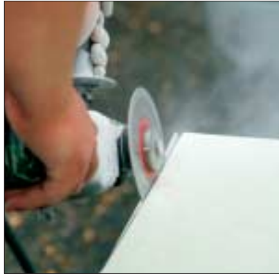
Installers make the final cuts on site to ensure a tight fit. Diamond-coated blades are necessary to cut through the hard quartz.
