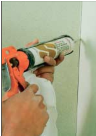
After all of the panels are installed, color-matched caulk is applied at all joints. The result is a watertight installation that requires very little maintenance.
