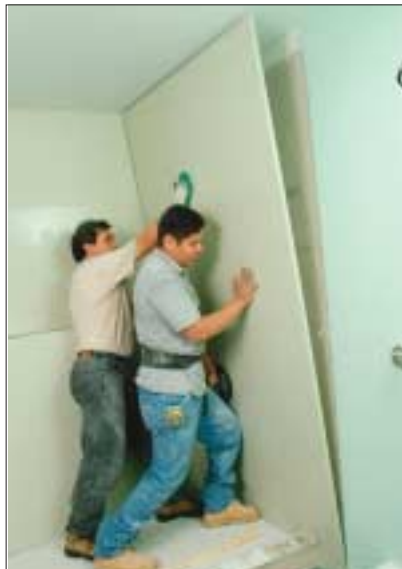
A special adhesive is applied to the backs of the panels; then they're pressed into place and braced in position while the adhesive cures.
