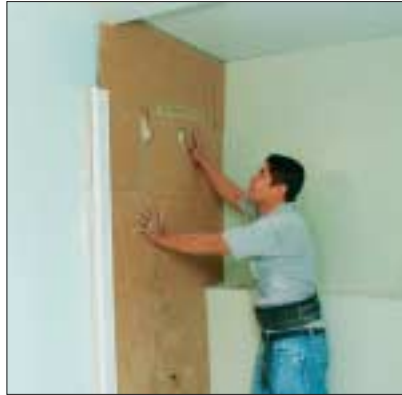
The first step in a typical installation (a shower surround is installed here) is to make cardboard templates of the areas so that the panels can be cut to rough size at the factory.
